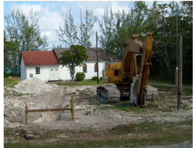
Mastic Point Church with construction going on in front of the building
